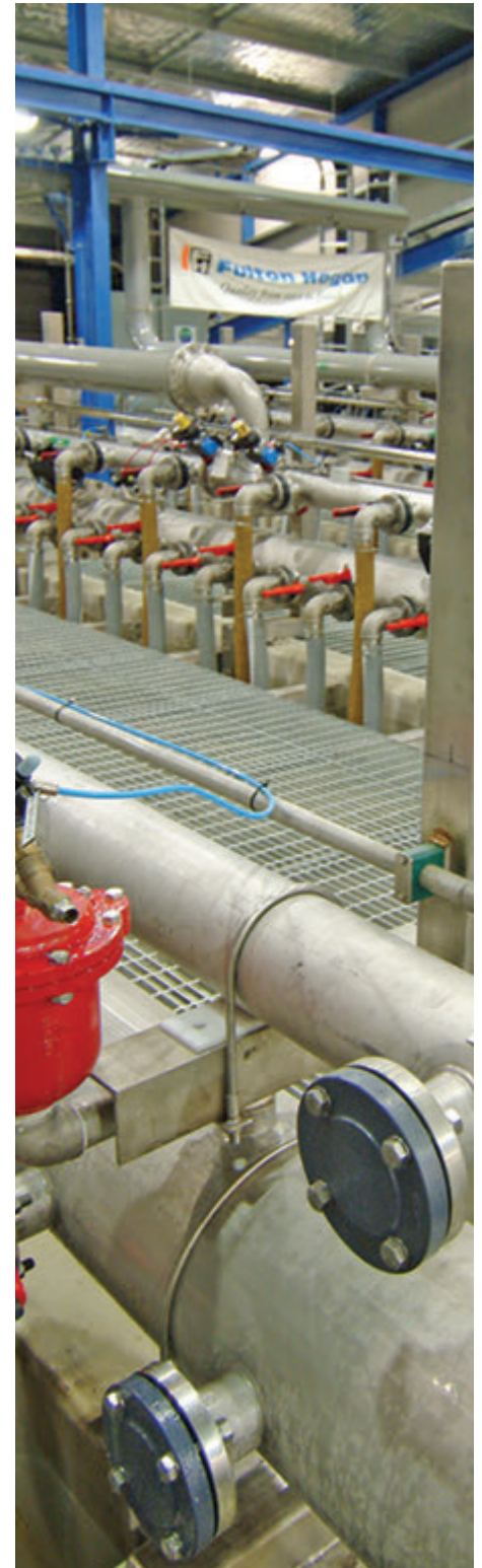
Inside the Nelson water treatment plant.
