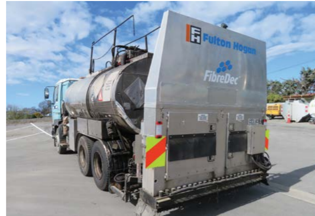
A truck-mounted 8,000-litre sprayer that blows fibreglass fibres in a membrane sandwiched between two layers of polymer modified emulsion
