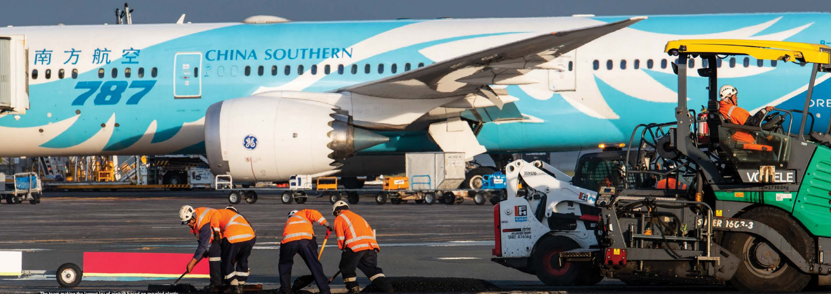
The team making the largest lay of asphalt based on recycled plastic
