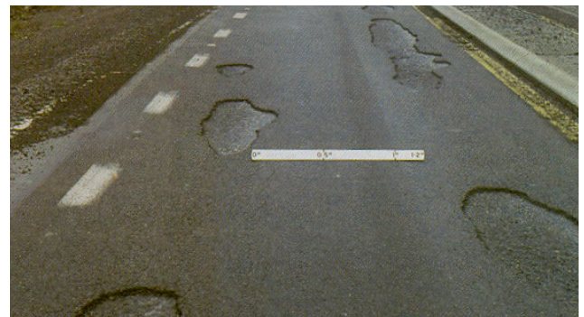
The high tyre pressures and heavy wheel loads from aircraft braking can result in delaminations in pavements constructed with traditional tack coat.
