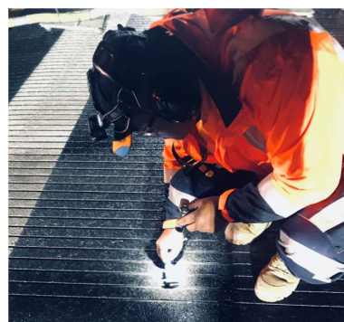
Quality control: Fulton Hogan is testing the groove dimensions and alignment during grooving operations
